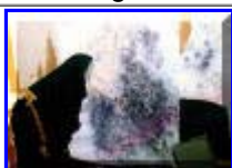
Mold growth behind wallpaper
