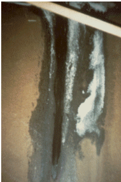
Stachybotrys (dark area) as found on drywall.
